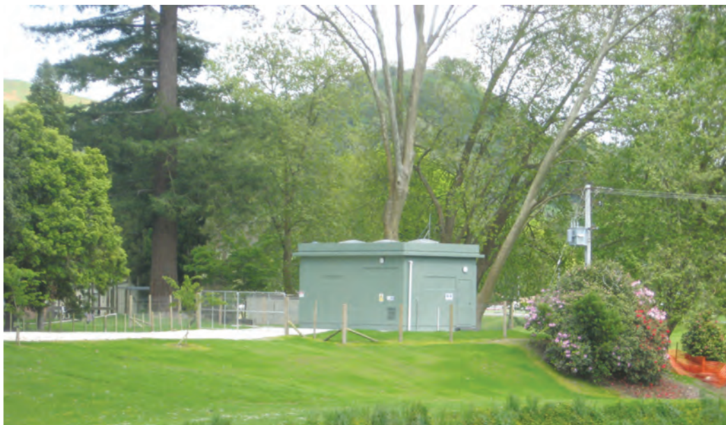
Te Kuiti Pump Station
